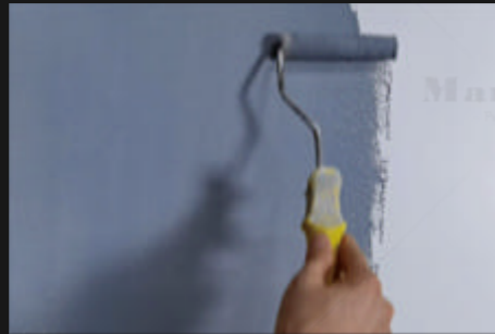
③ With the model of "TCF", which shall be the sealing primer. Brush them which shall be completely waterproof.
